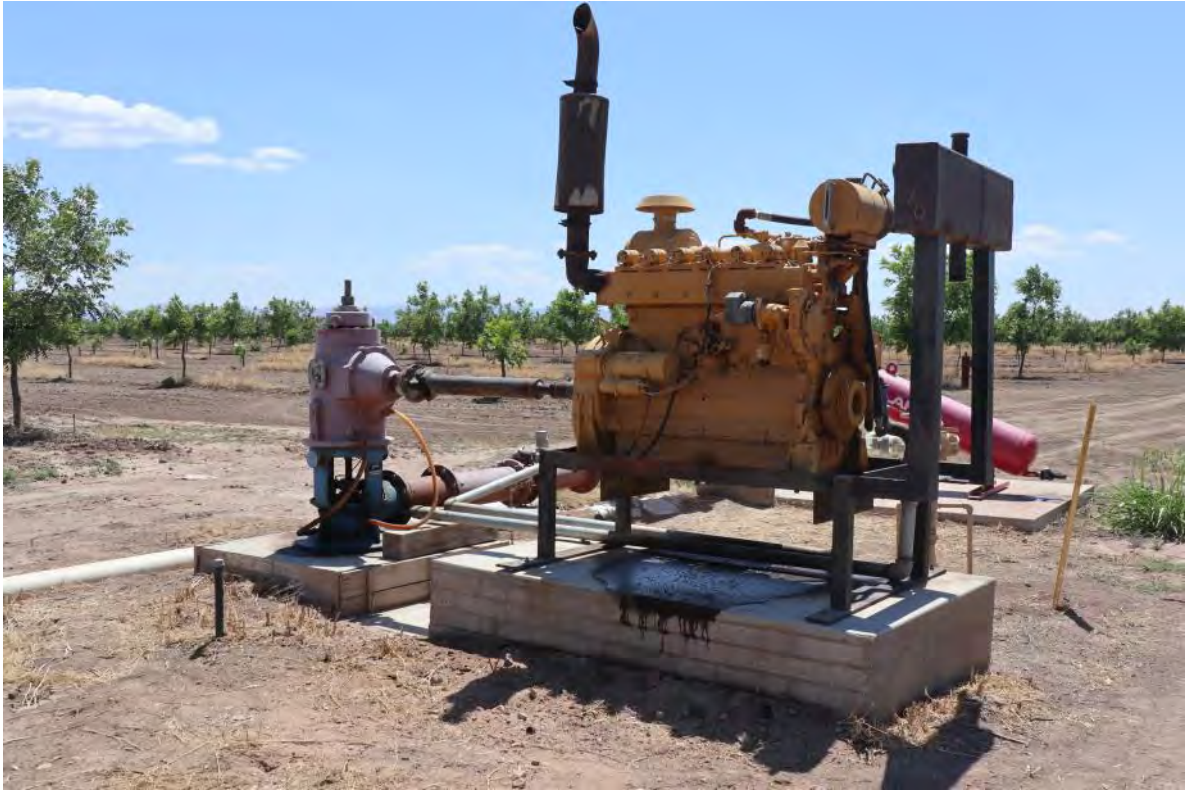
Natural gas driven irrigation pump
