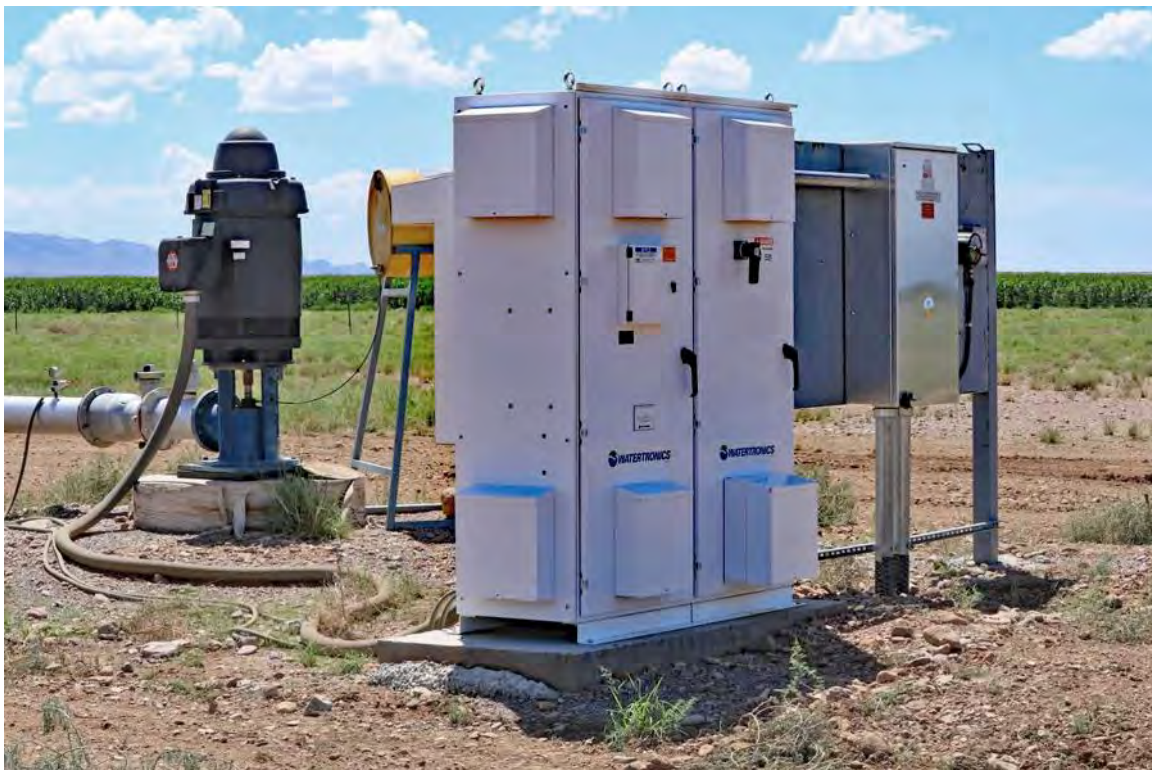
Well No. 1, drilled 2/24/20, 1090' deep, 250 hp, 1,000 GPM
