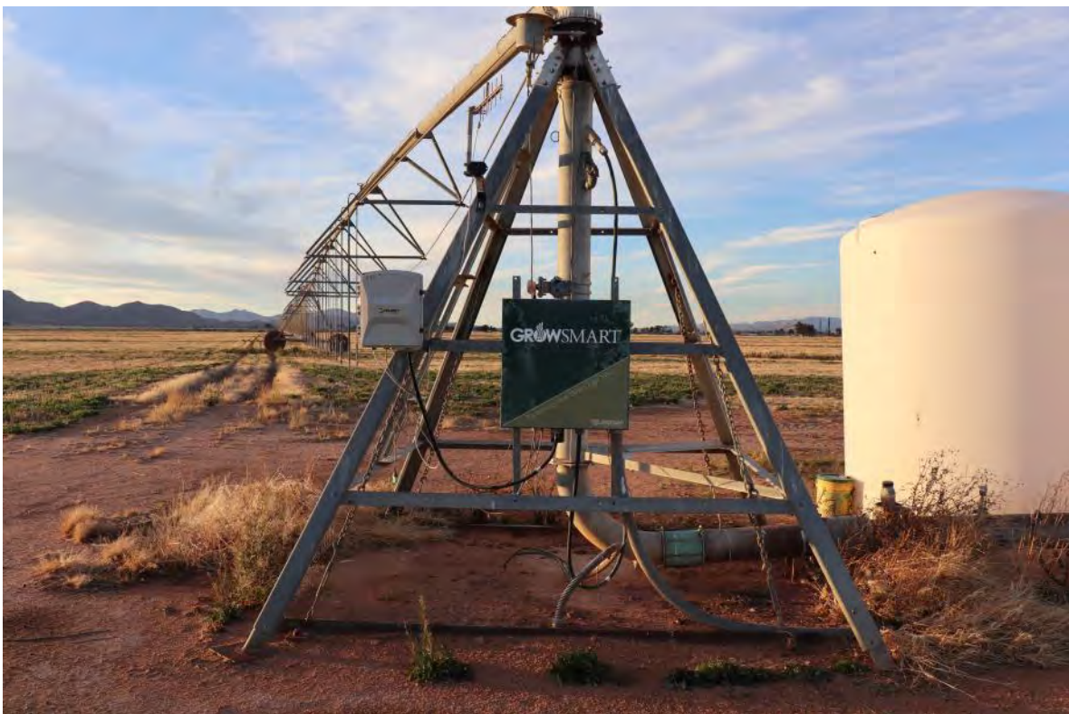
Growsmart control panel
