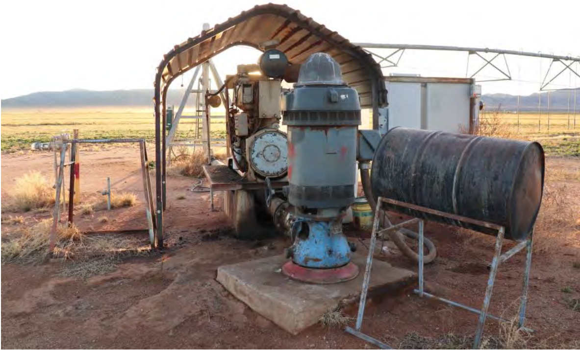
Turbine pump, electric motor with gas engine backup
