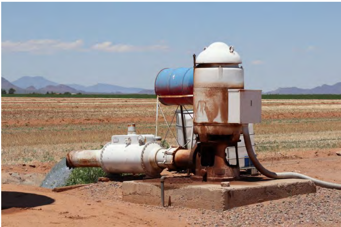
Well no. 1, 1300' deep, 16" casing, 250 hp., 1,100 gpm
