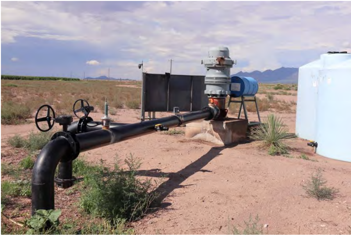
Well No. 2, 810' deep, 200 hp electric motor, approx. 800 gpm
