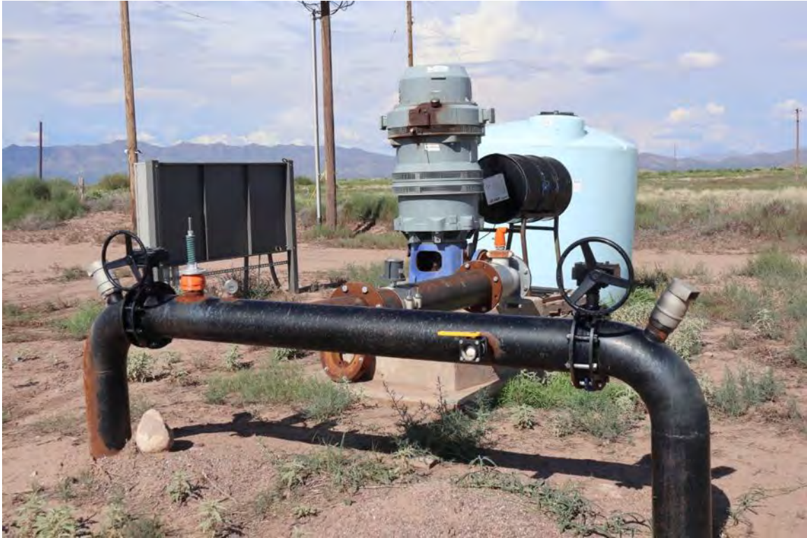
Well No. 3, 1,045' deep, 200 hp electric motor, approx. 800 gpm
