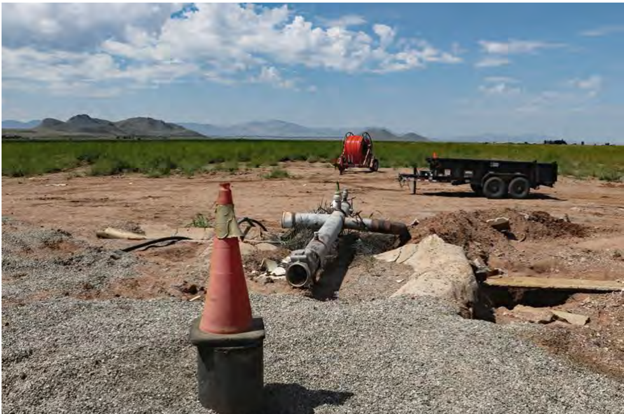
Recently improved irrigation well. (August, 2021); deepened to 1,000' with 12" casing.
