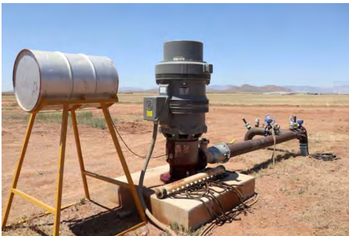
Irrigation well 500' deep, 150 HP, 675 GPM
