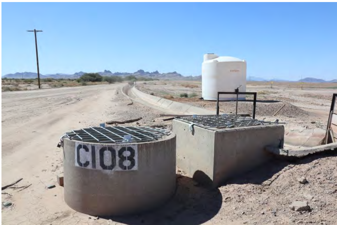
Irrigation district turn-out, CAIDD C108
