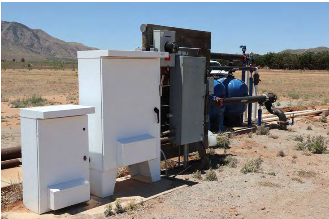
Well 915' deep with submersible pump, 250 gpm
