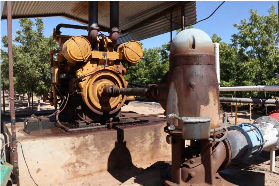
700' well, Cat natural gas engine, 1,500 GPM
